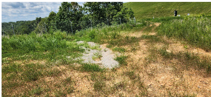
Road and Grassy Area Erosion
