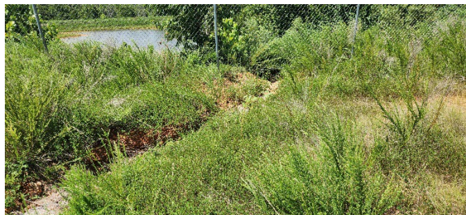
Grassy Area Erosion
